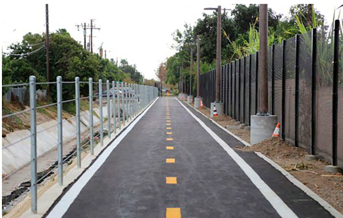
Santa Ana Gardens Flood Control Channel Bikeway
